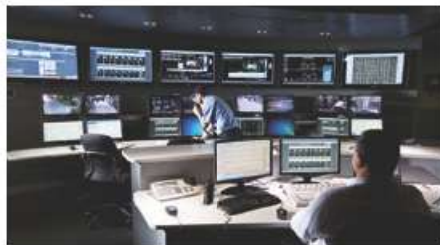
Command and control center
