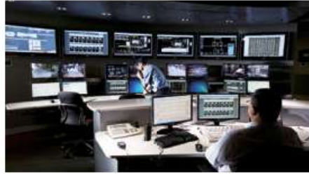
command and control center
